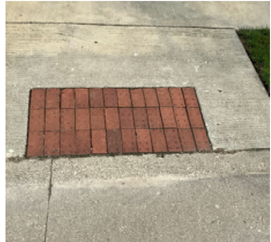
Example of DW with visual contrast but sheared tactile domes and lacking full width
