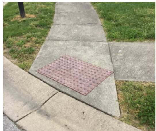
Example of lack of level turning space at corner
