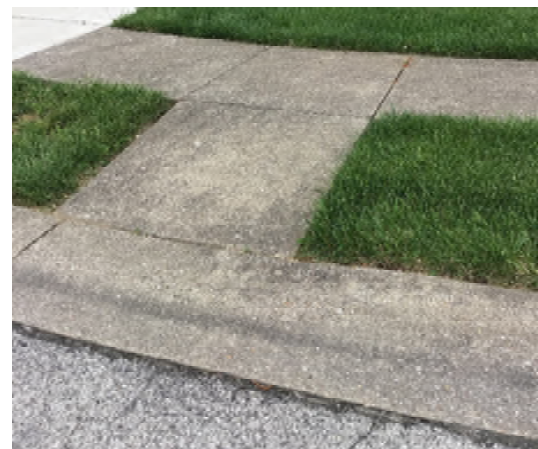
Example of displacement where pavement meets gutter
