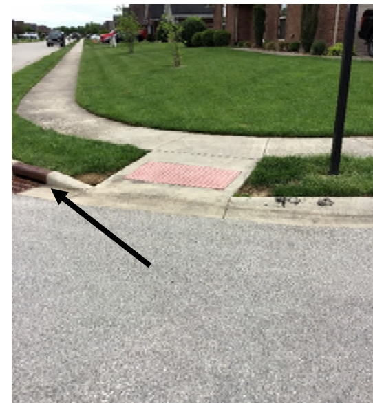
Example of drainage structure located near ramp, creating potential for drainage concerns.
