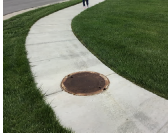
Example of potential manhole obstruction if displacements occur as infrastructure ages, or pickholes exceed allowable dimensions.
