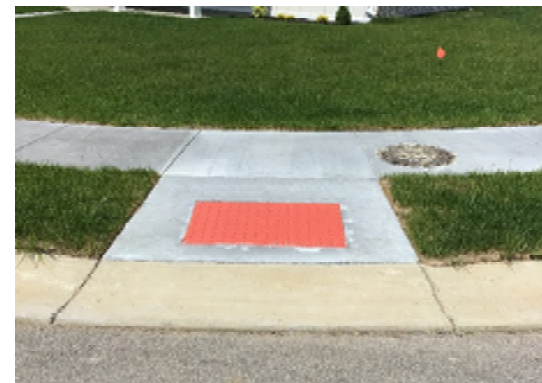
Example of DW that does not extend full width of curb ramp and is too far from back of curb
