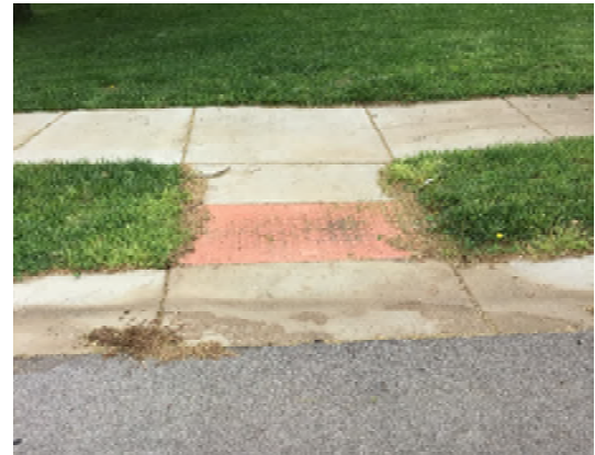
Evidence of sediment build-up indicative of a drainage issue
