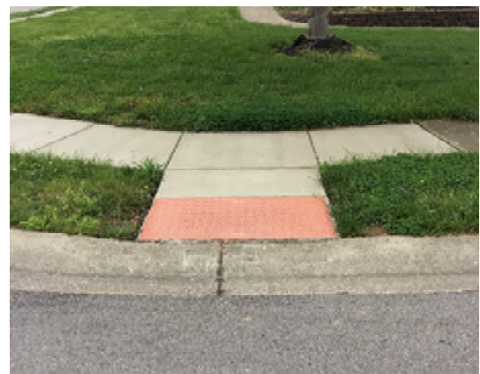
Rolled curb creates non-compliant level change
